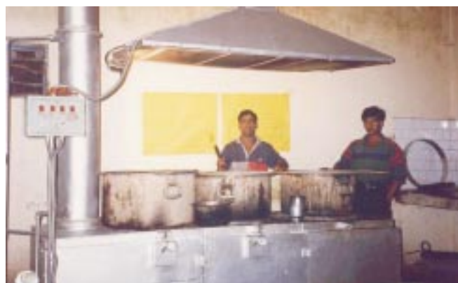
Solid Biomass Fired Furnace
