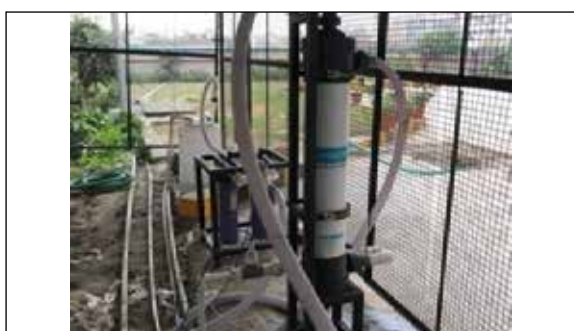
Sewage treatment plant based on UF Membrane of PAN
